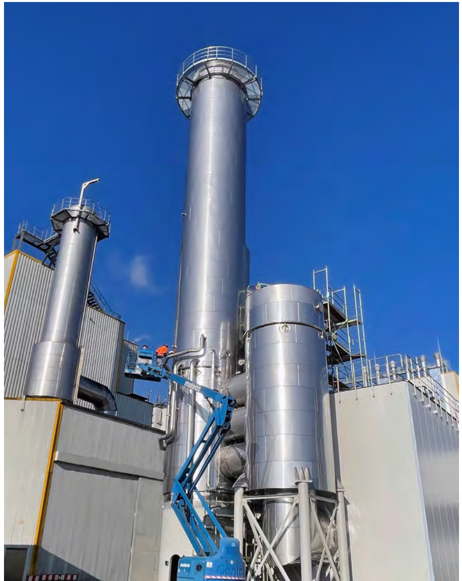
The final touches on the evaporator at our customer Jäckering in Hamm. On the left, the preliminary project realized in 2016.
