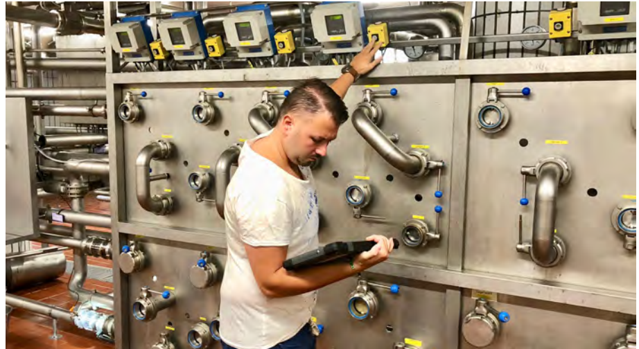
The process events can be directly monitored through the nearby operator station.
